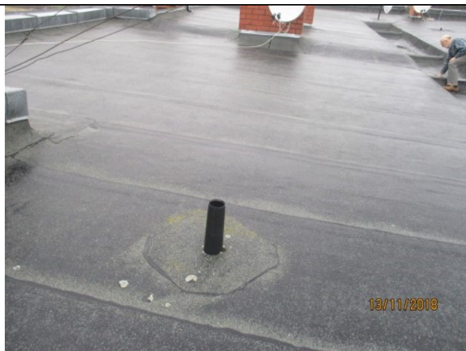
4.8.6. att. Aerators bez nasegcepures
